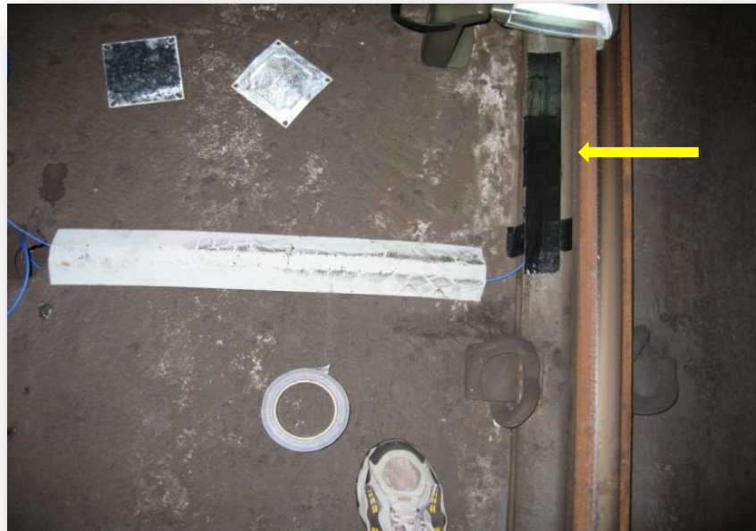
FBG strain sensor installed on the track.
